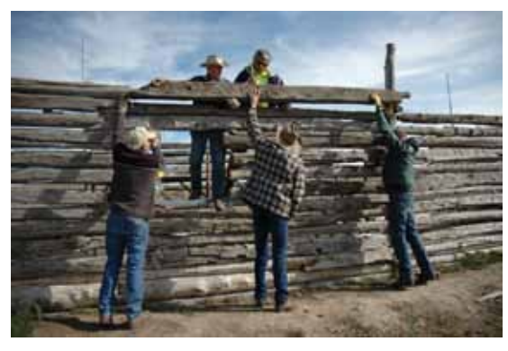
GPNPS members at work restoring the cabin. Photos courtesy of Gallatin Valley Native Plant Society.
